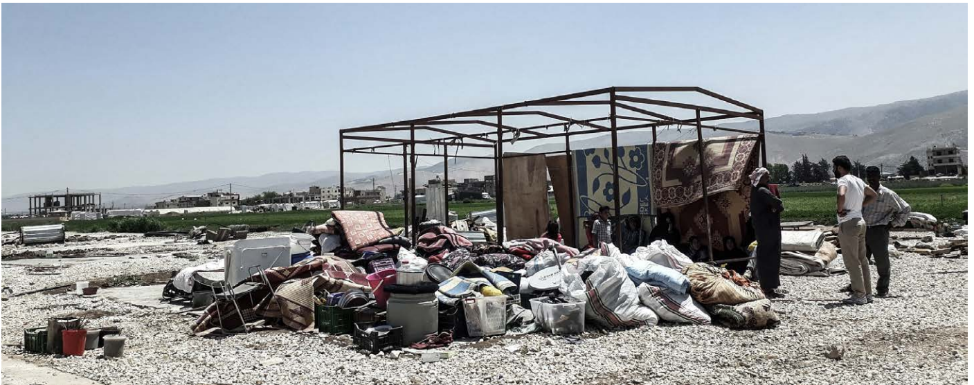
The dismantling of the settlement on Nawfal Ahmed Saad's land outside Dalhamiye, Lebanon in May. Photo courtesy of Refugees Deeply/Abby Sewell
