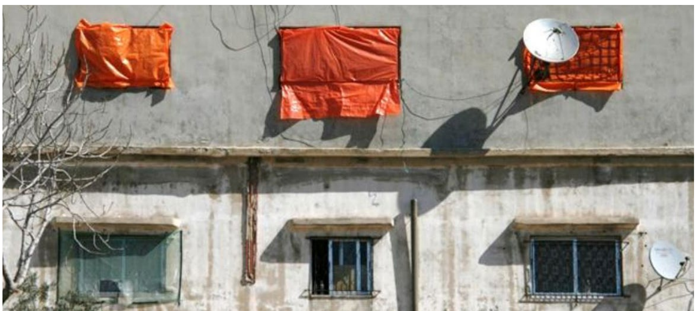
Tarpaulins are used to seal the windows of an unfinished building home to Syrian refugees in Mafraq, Jordan, Credit: REACH
